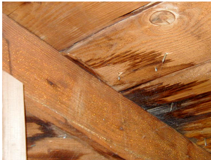
Staining on roof sheathing at the roof edge
