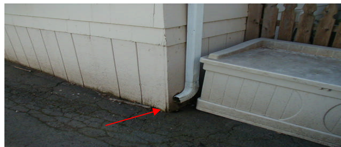
Inadequately diverted downspout
