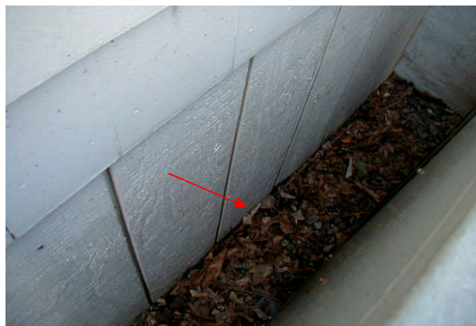
Plywood in contact with soil surrounding a crawlspace
