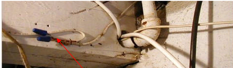
Hazardous Electrical Connections
