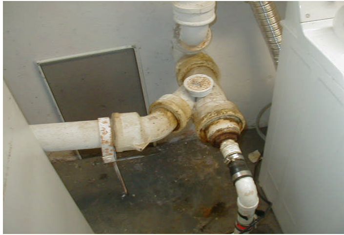
Sump pump discharging into drain plumbing
