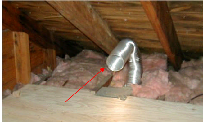
Improper Venting into the Attic
